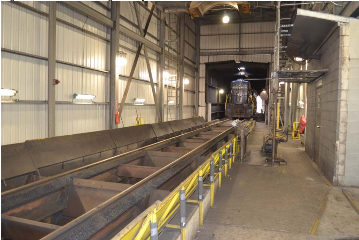
Figure 3: Coal Off-loading Facility
